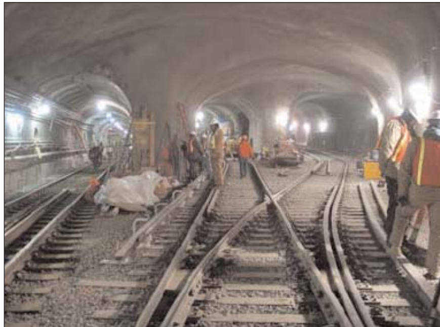
The Port Authority is creating new crossover tracks at Exchange Place in Jersey City to enable PATH service restoration at that station by June 2003.
