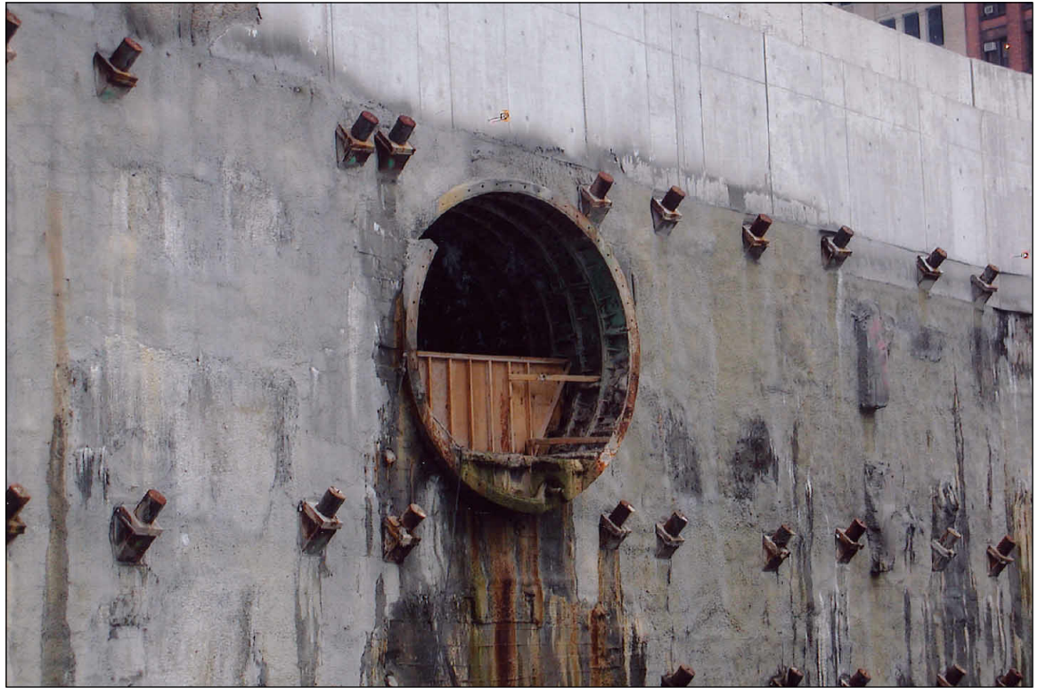
East slurry wall, view of Hudson Tube
