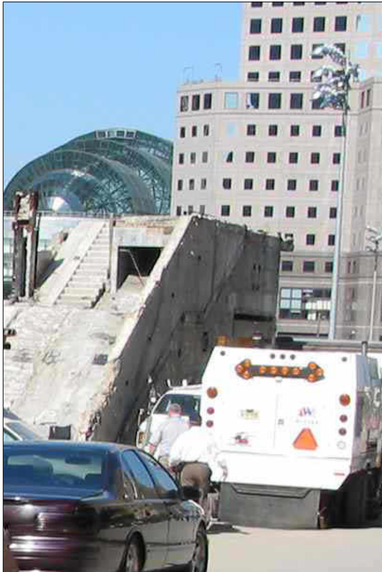
View of damaged stair and escalator structure on Vesey Street
